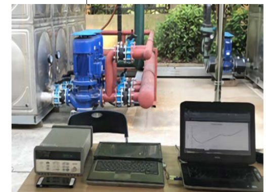
Cooling tower thermal performance test
